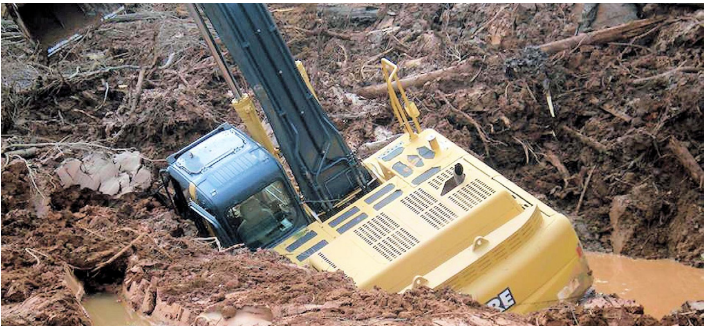
Figure 2: If this excavator had sent warning alerts back to the equipment rental firm, perhaps the rental manager could have intervened before too much damage was done.
